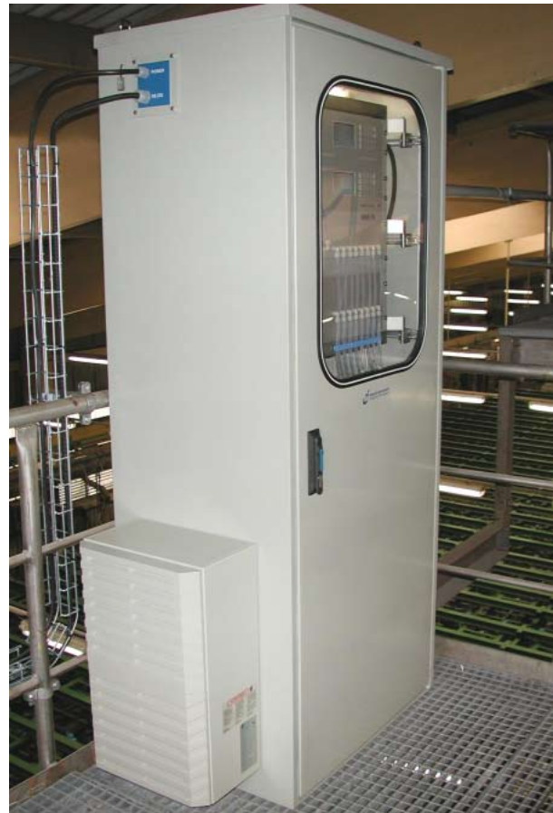
MMS: Installation of a 16-channel MMS in a chlor-alkali plant for cellroom monitoring
